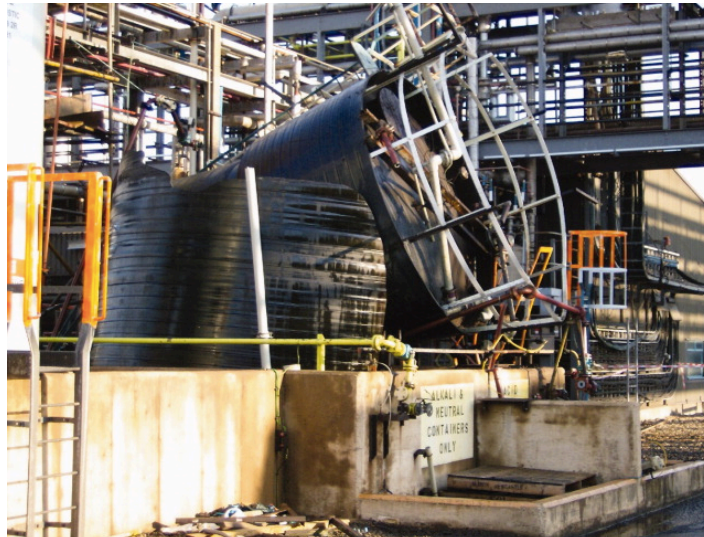
(Figure of ruptured tank)
